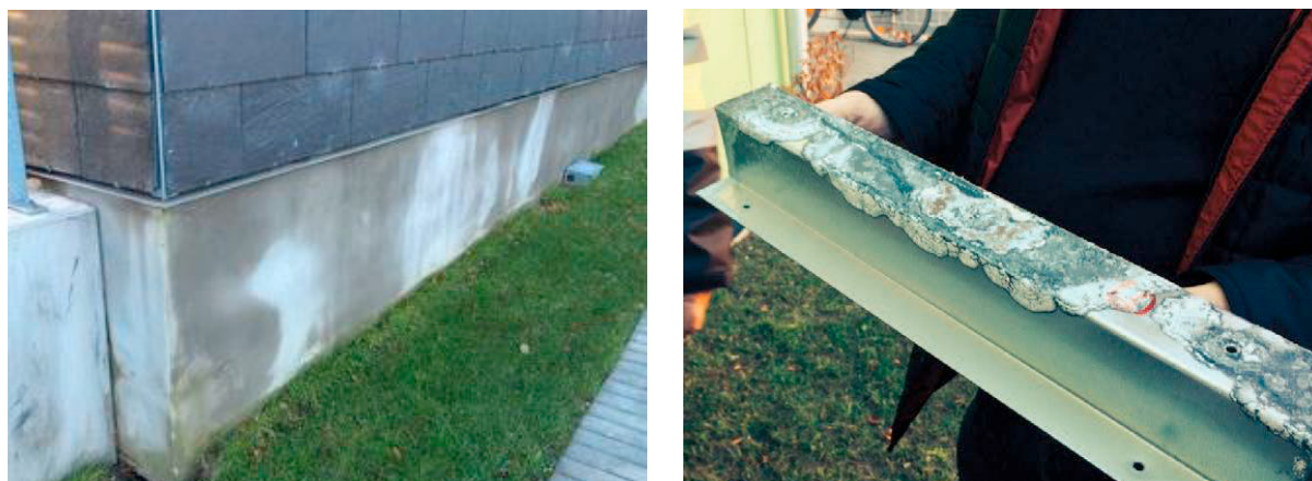
Fig. 3. (a) Water drops containing chloride ions run down the vertical MgO-boards and drain out of the wall from behind the wall's siding boards; (b) Zink covering of the steel profile is corroded as a result of direct contact with salty leaked water from the adjacent MgO-board.
