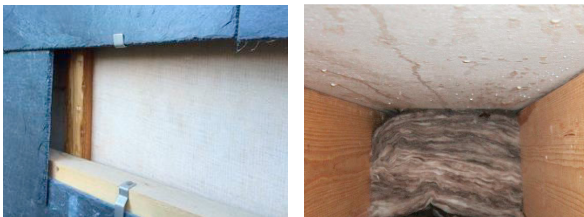
Fig. 2. (a) The MgO-board is placed facing the air gap, which is behind the siding boards made of natural slates; (b) Salty water drops on a vertical MgO-board on the side that faces the insulation filled cavity inside the wall.
