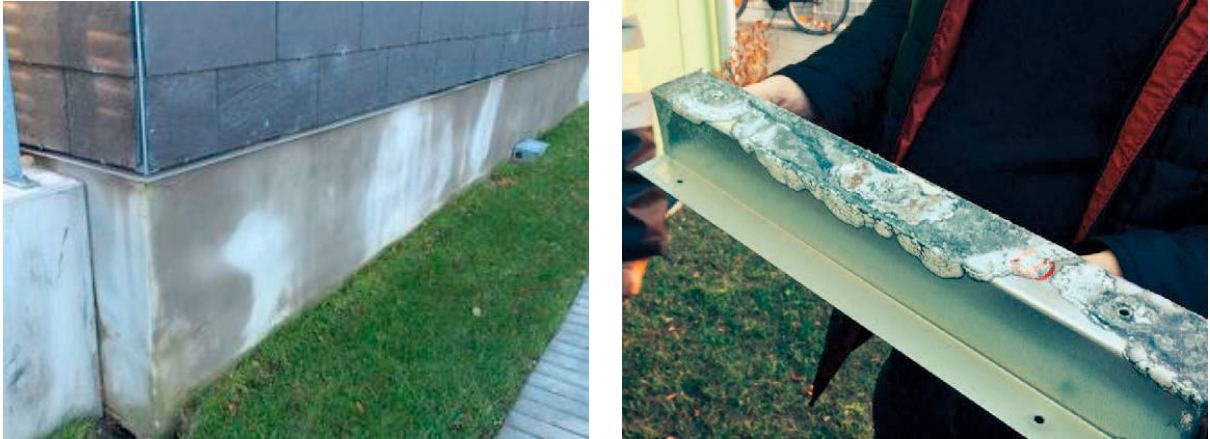
Fig. 3. (a) Water drops containing chloride ions run down the vertical MgO-boards and drain out of the wall from behind the wall's siding boards; (b) Zink covering of the steel profile is corroded as a result of direct contact with salty leaked water from the adjacent MgO-board.
