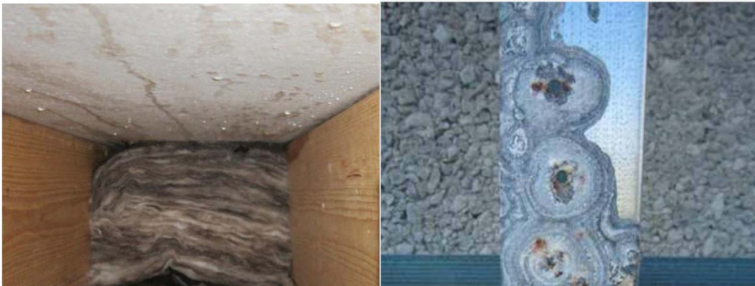
Figure 2-1-Evidence of damages due to MgO boards: Leachate visible on MgO board due to excessive moisture absorption (left) and corrosion of contacting metal framework (right) Source: (Hansen et al. 2016)
